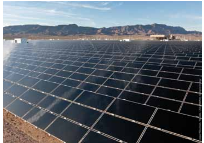
58-MW photovoltaic installation at Copper Mountain, Nevada
